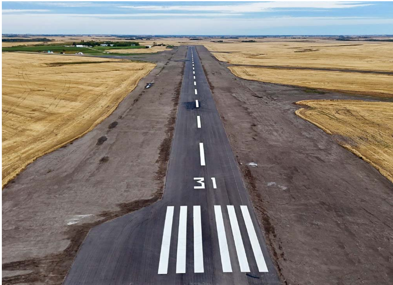
The new, completed runway at Moosomin airport. The runway had the lines painted on it on September 14 and 15. The airport expansion includes a 5,000-foot by 75-foot paved runway, along with a new taxiway and apron, which were completed this summer.
