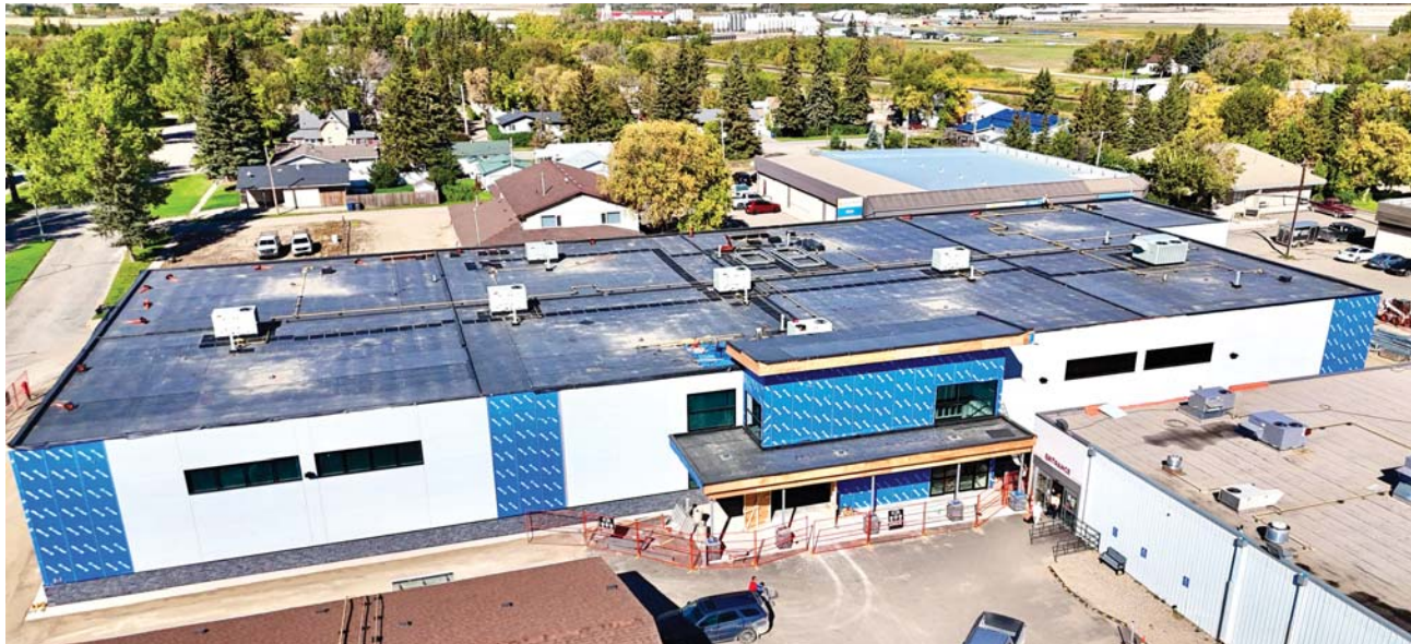
Work continues on Borderland Co-op's 30,000 square foot grocery store in Moosomin. When the new store is complete, the current grocery store will be demolished.
