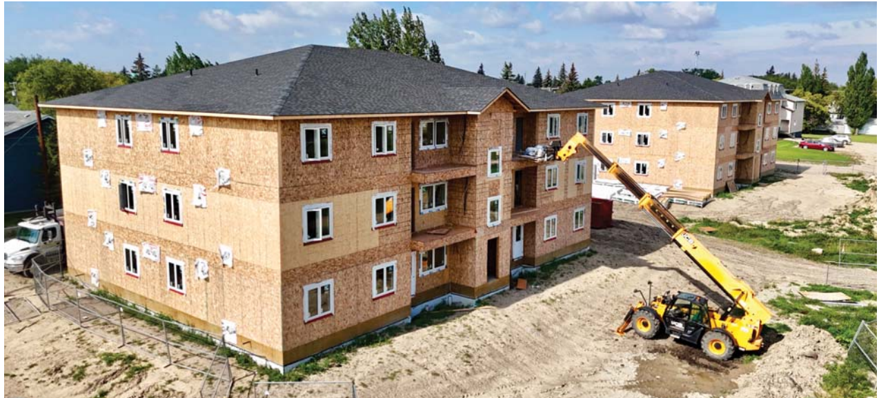
Keller Developments has two apartment buildings under construction in Moosomin that will benefit from the community's new residential construction housing incentive. (Kevin Weedmark photos)
